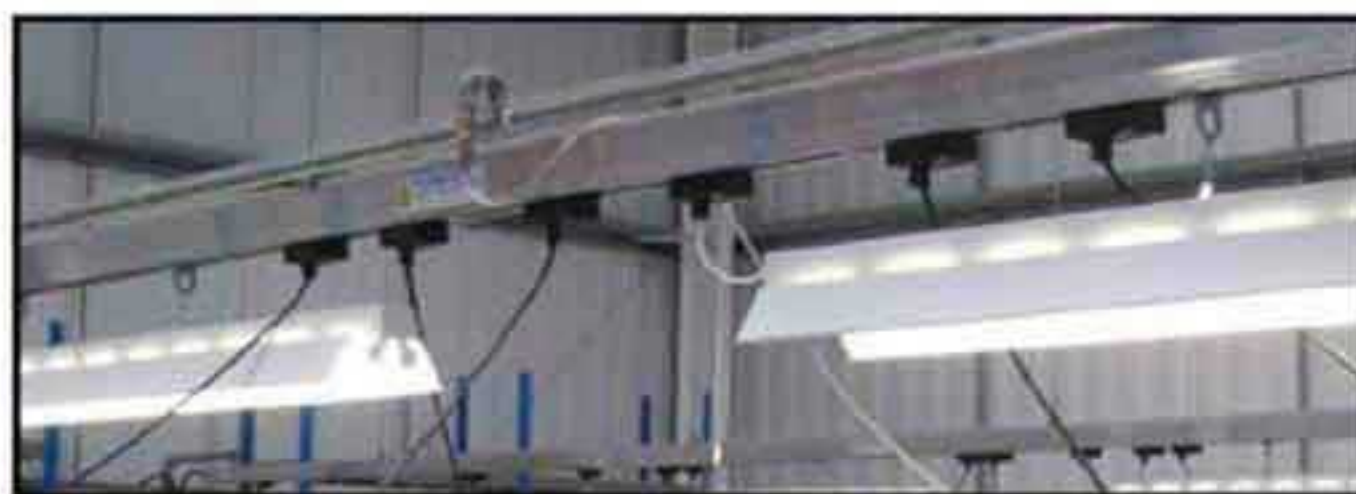
Typical Plugway installation for garment production
